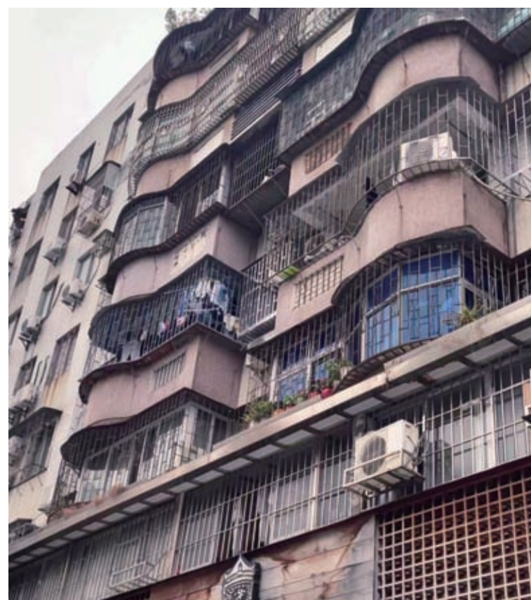
Caged balconies in an old neighborhood in the southern city of Shenzhen limit access to sunshine for clothes drying. — Ti Gong
